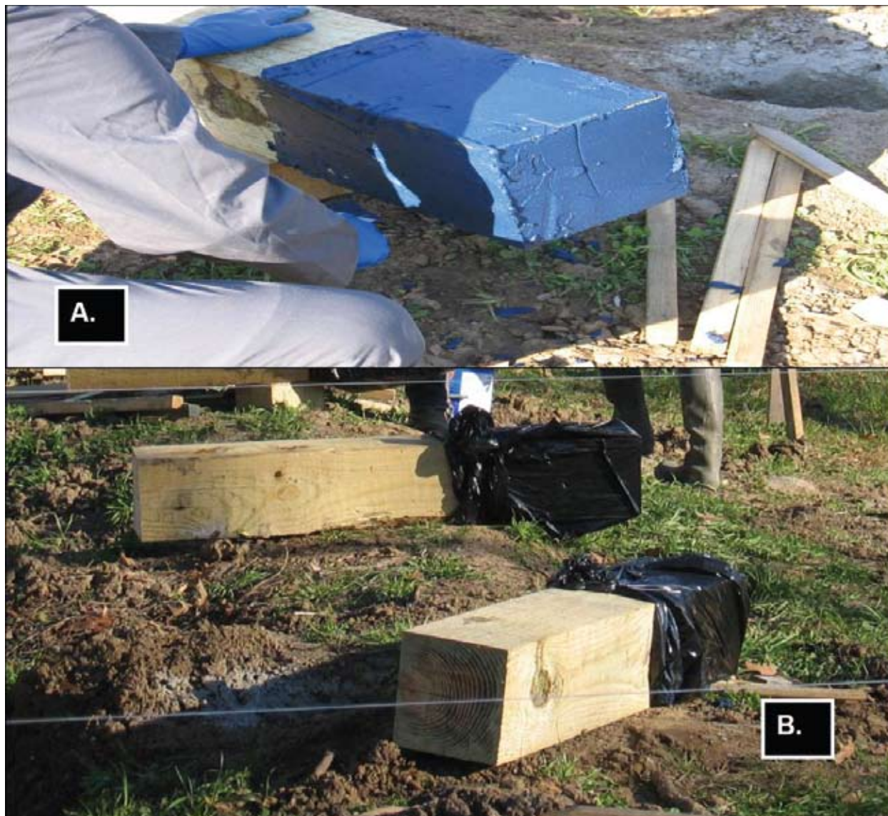
Figure 7. Treated wood columns (posts) used as either structural supports for deck surfaces or railings, if cut to expose new wood, should be installed with the original end oriented toward the soil and the freshly-cut end oriented upward. (A.) the original treated end of the treated column was treated with a copper-boron paste (CuWrap 20) as a supplemental treatment before installation (B.) the treated end was covered with plastic to encourage diffusion and protect the treatment from the environment (a hole was cut into the bottom of the plastic to allow moisture to drain).
