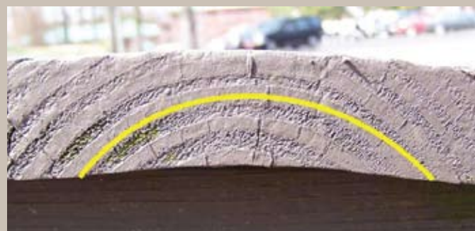
Figure 1. A cross section of an older decking board showing the grain orientation bark side up, Bark side up orientation will help reduce weathering-related defects.
