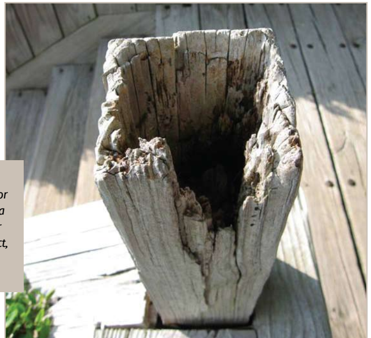
Figure 5. A cap (circle) or railing board (arrow) should cover exposed end-grain of wood, after treatment with a water-repellent preservative, to deter moisture from pooling on the end-grain of the wood.
