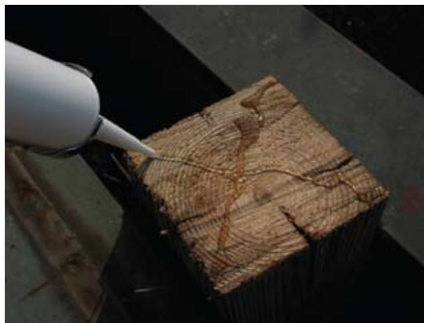
Figure 11. (A.) A viscous borate solution being applied to the top of a deck railing post before it was covered by a galvanized top.
