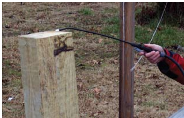
Figure 9. Water repellants can be applied by spray or brush to the top of support posts to protect them from moisture and decay.
